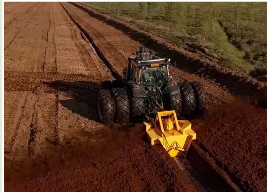
Field Drain Construction with Typical Profile of 1.5m x 1.5m at ~33m Intervals
